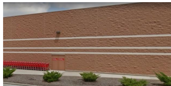
Larger bricks or concrete masonry units (CMUs) with color and texture can be appropriate for “big box” or larger buildings.
